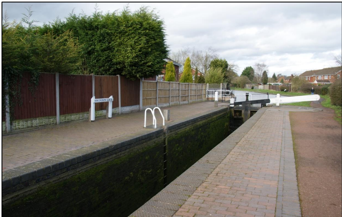
Figure 5.3. Swindon lock, S&W canal, looking north to Marsh Lock showing the 500-yard towpath diversion visible on the right – the only towpath change in a 15-mile section. Photograph taken from the Swindon Road turnover bridge.
