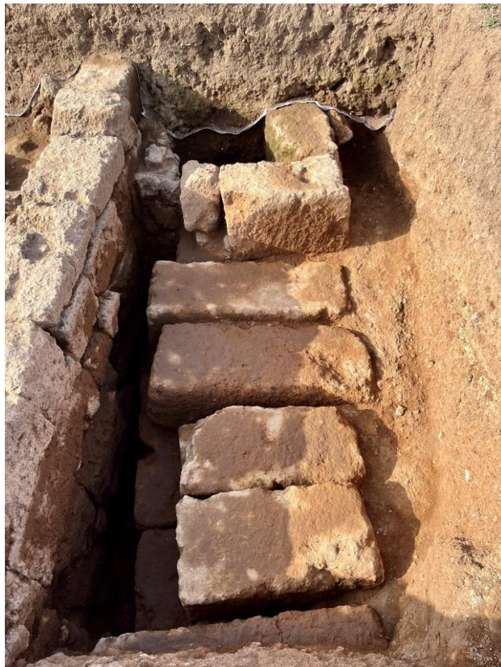
Fig. 7. Large drain feature running below Room I.7 in building north of macellum, view from north showing large tuff blocks forming top of drain and vertical feature at south.
